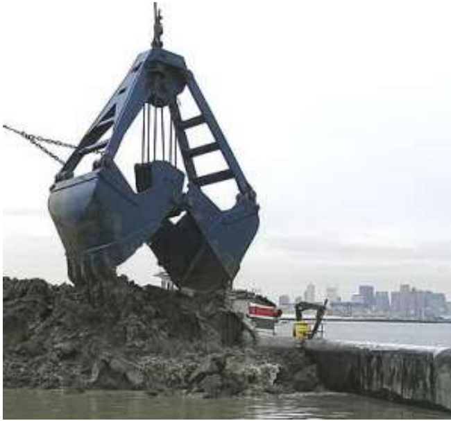
Figure 5 – On the left, a mechanical bucket dredging showing consolidated material, and on the right, the hopper of a dredge showing a slurry of dredged material
